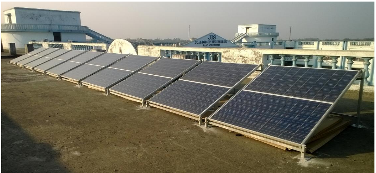
5 kw on grid solar power plant at JIS College of Engineering Campus
